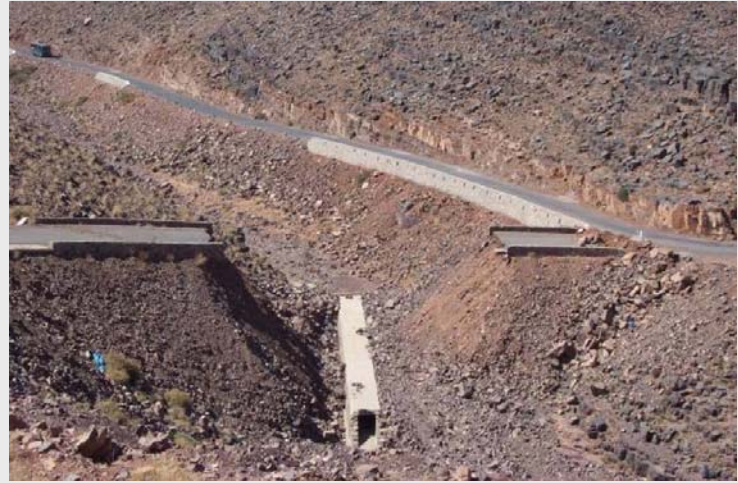
Destroyed bridge in the Anti-Atlas Mountains
